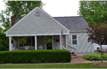
Address 255 N. Rating C Year 1950 Style American Small House Notes Extensive remodeling/new porch, retains proportional shape
